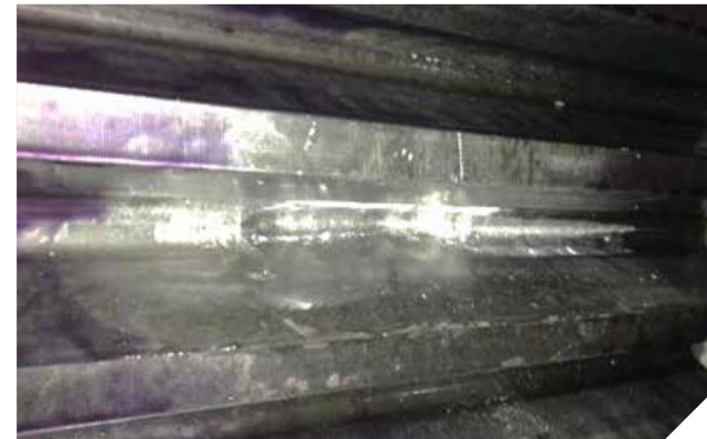
Once detected, cracks are assessed and treated immediately by OEM experts
