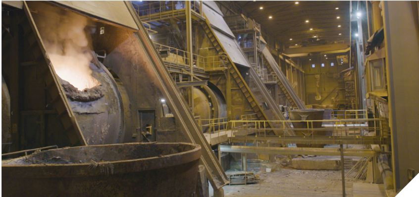
The Metso Outotec Converter Hood System installed at Boliden Rönnskär Smelter
