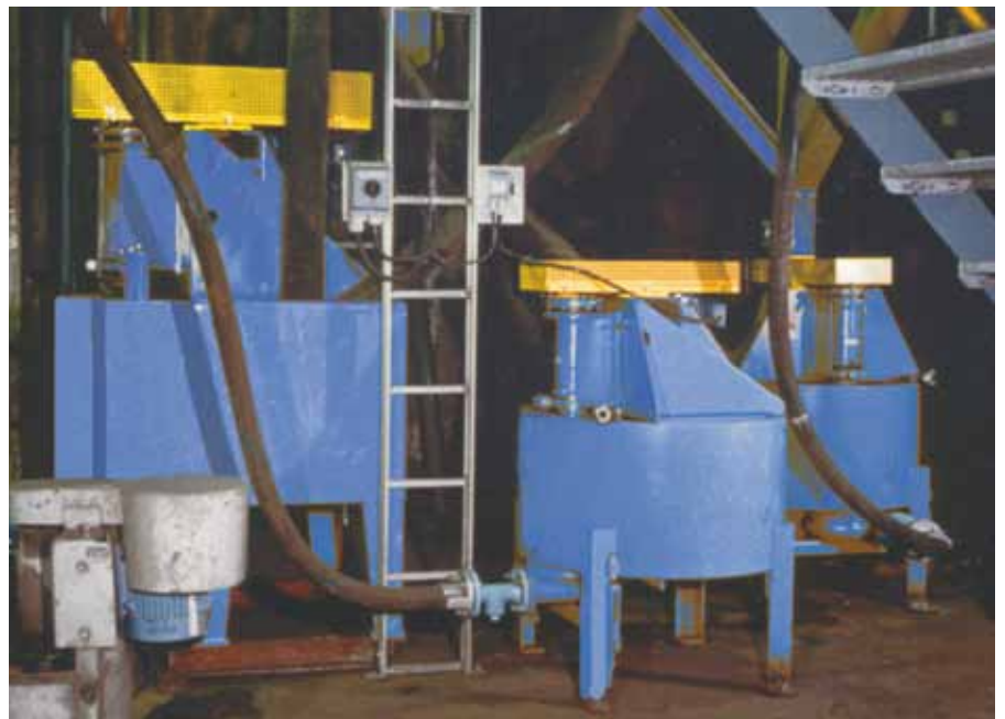
Metso VT pumps for pumping of concentrate, middlings and tailings from spirals for treatment of slag <2 mm.
