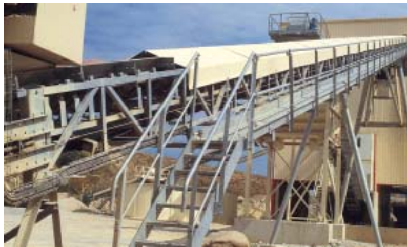
Conveyor with side walkway and cover.
