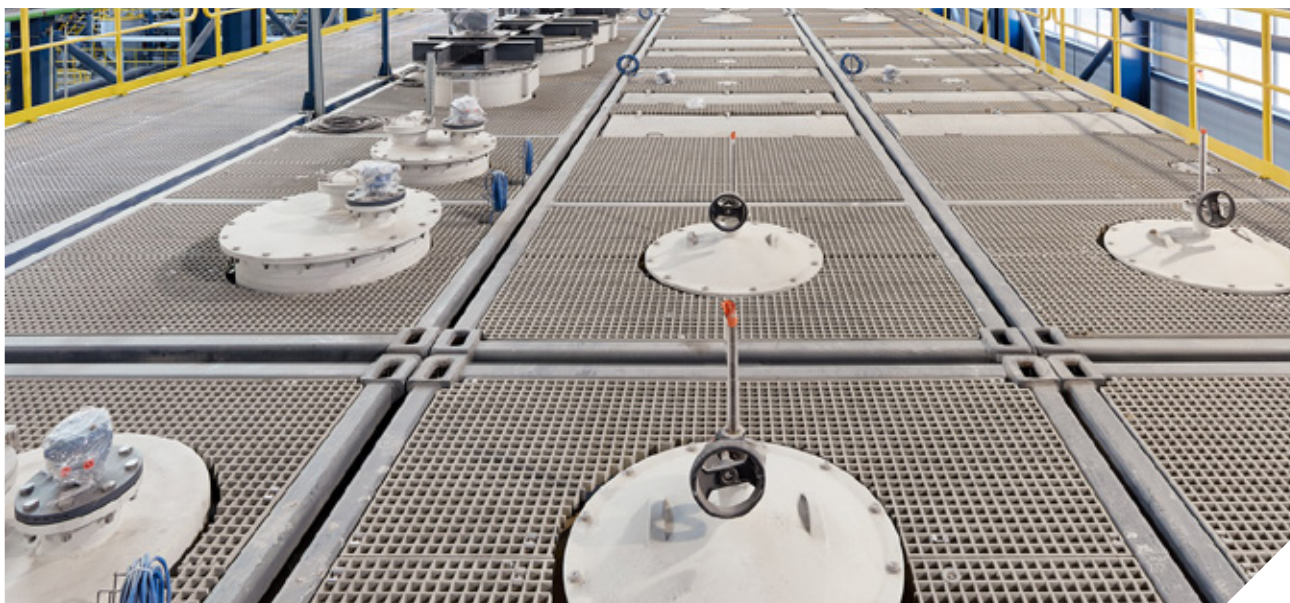
Modular VSFX solvent extraction plant
