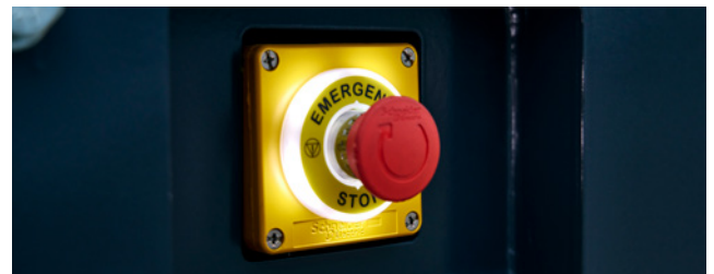
Figure 9: Emergency stop station
