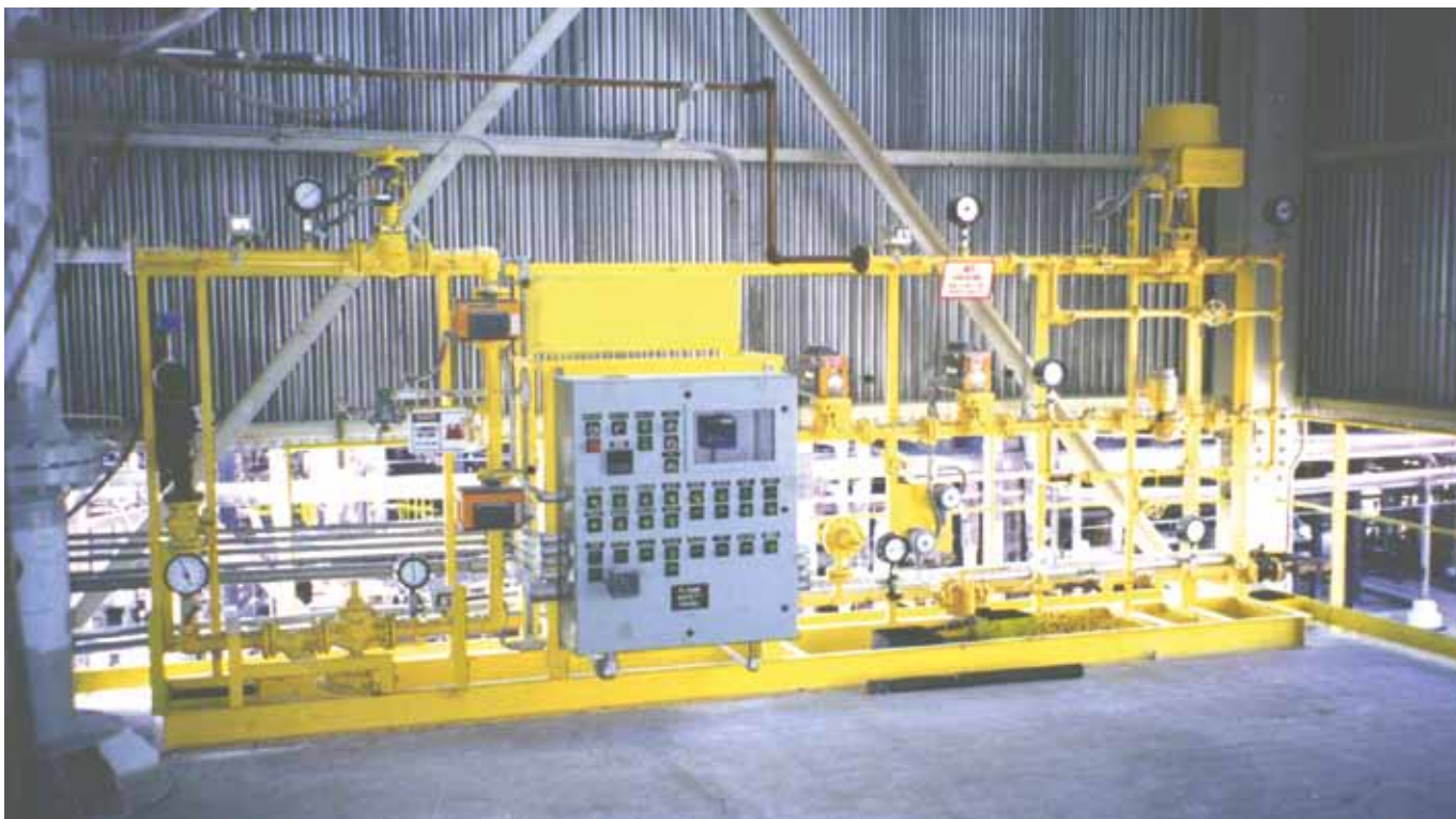
A typical gas valve train
