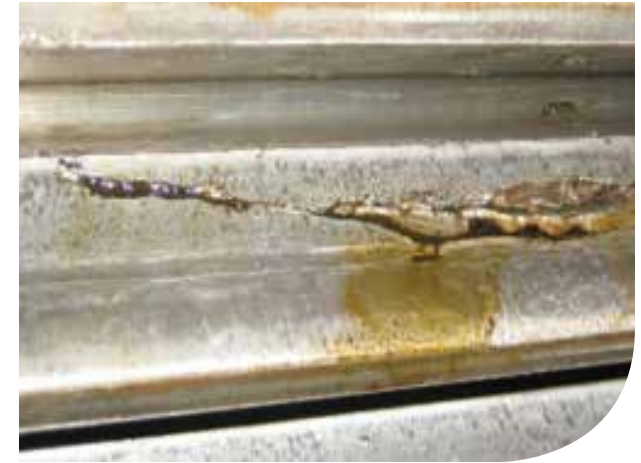
Mill Comprehensive/Customized: A crack and severe damage found on a gear tooth while performing a pinion and gear MPI.
