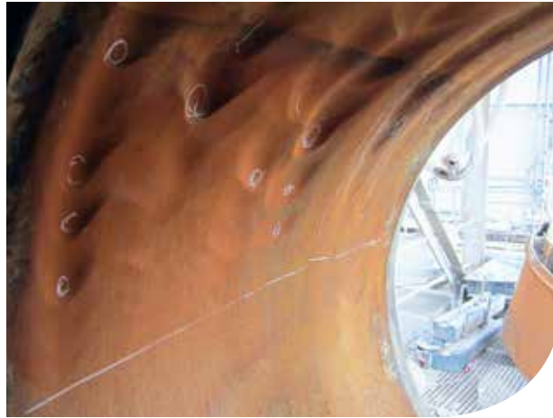
Mill Mechanical Verification: Wash pockets discovered inside the mill trunnions. These can be detected from the outside through UT.
