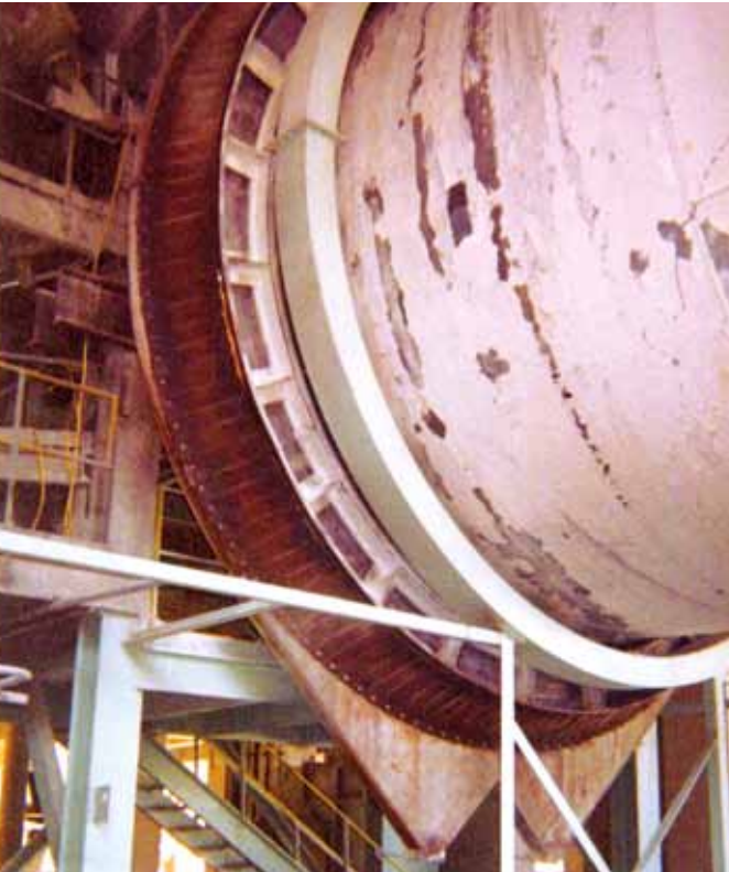
Superdeal seal installed on the feed end of a cement kiln
