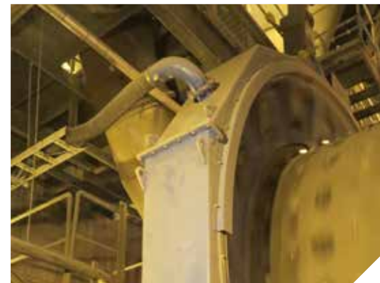
Protecting the gear with a pressurized guard
