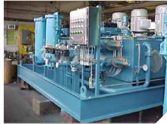
Hydrostatic lubrication system
