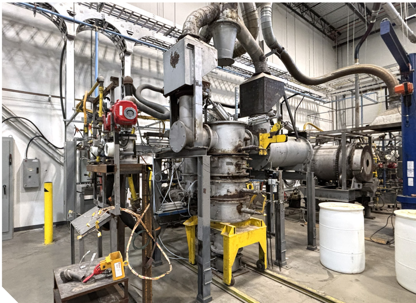
Figure 12: Pot grate system at the Metso York Test Center, Manchester PA USA
